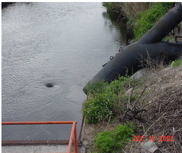
Figure 1: Surface water Vortex due to insufficient pipe submergence depth
