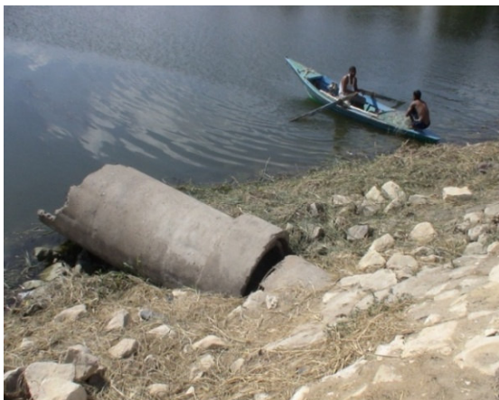
Picture (1) Broken pipes at Upstream
