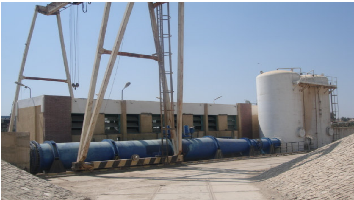
Figure (8) Anti surge vessels at El Batts pumping station
