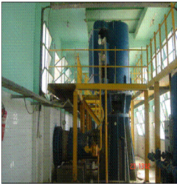
Fig. (1) Photograph of El Batts pumping units
