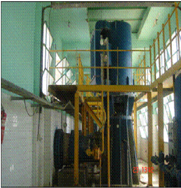
Fig. (1) Photograph of El Batts pumping units
