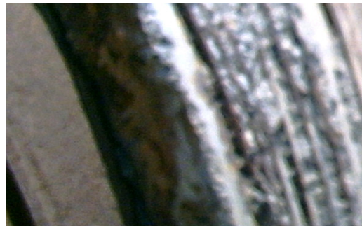
Fig. 4 Part of a corroded pipe
