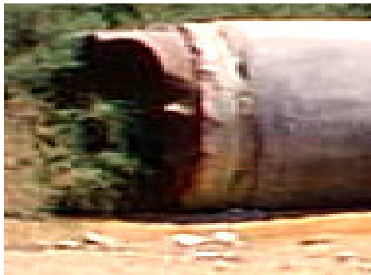
Fig. 7 Part of a corroded pipe
