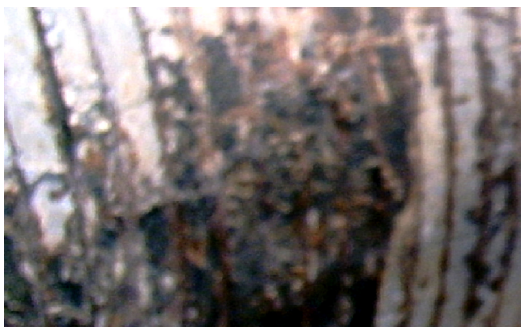
Fig. 3 Part of a corroded pipe
