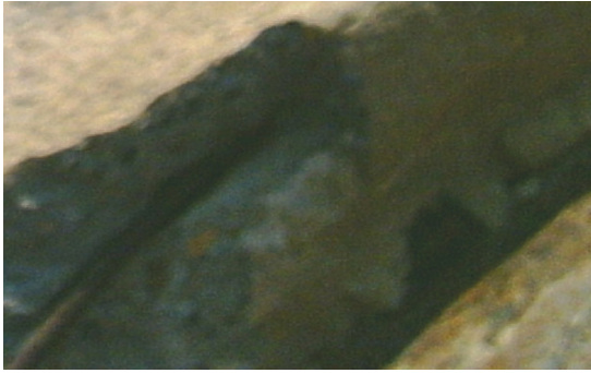
Fig. 5 Iron bars inside pipeline
