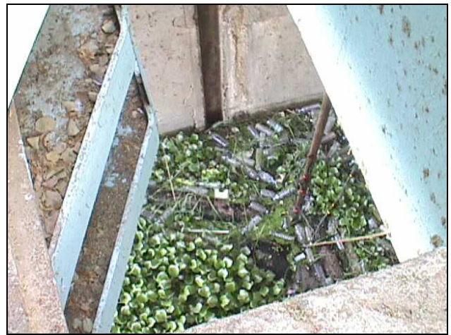
Figure (3) Photographs of Different Contaminants blocking Pump Intake
