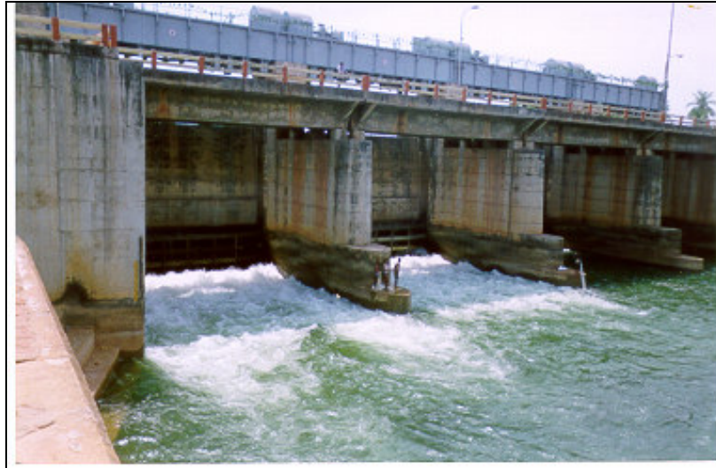
Fig. 8 Barrage Gates in Operation
