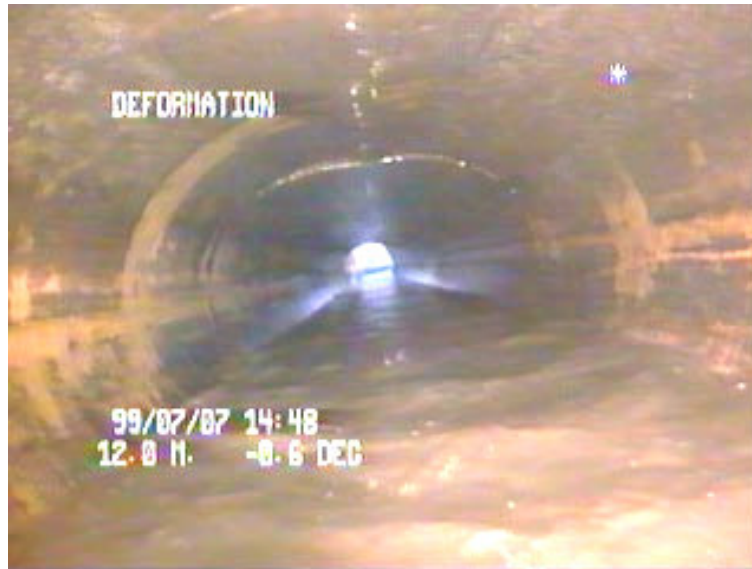
Figure 3 Deformation of the GRP Sewer
